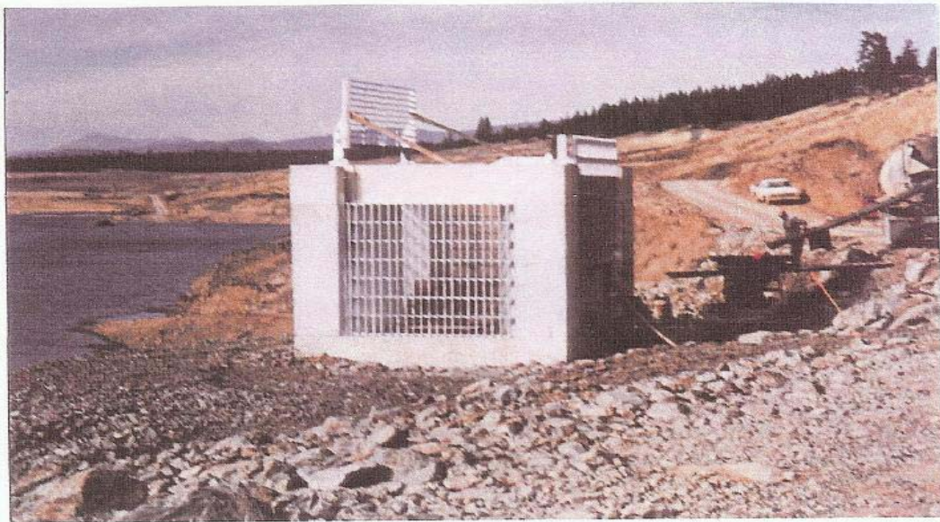
PHOTOGRAPH NO. II-5. MASON DAM, BAKER PROJECT, OREGON. Intake structure with hinged top trashrack.
